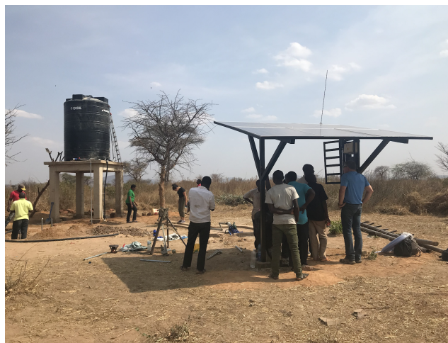
The solar powered pump and local tank
